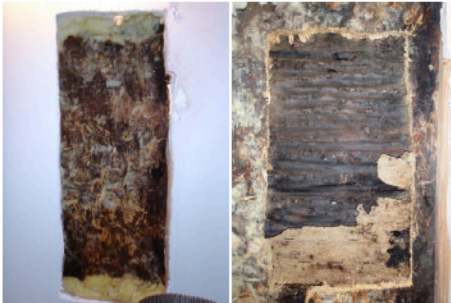
Figures 2 and 3: Master Bathroom – South Wall Destructive Testing – Water-Staining and Probable Visible Mold to Exterior OSB Sheathing (left) and Water-Stained and Degraded Building Paper (right)
